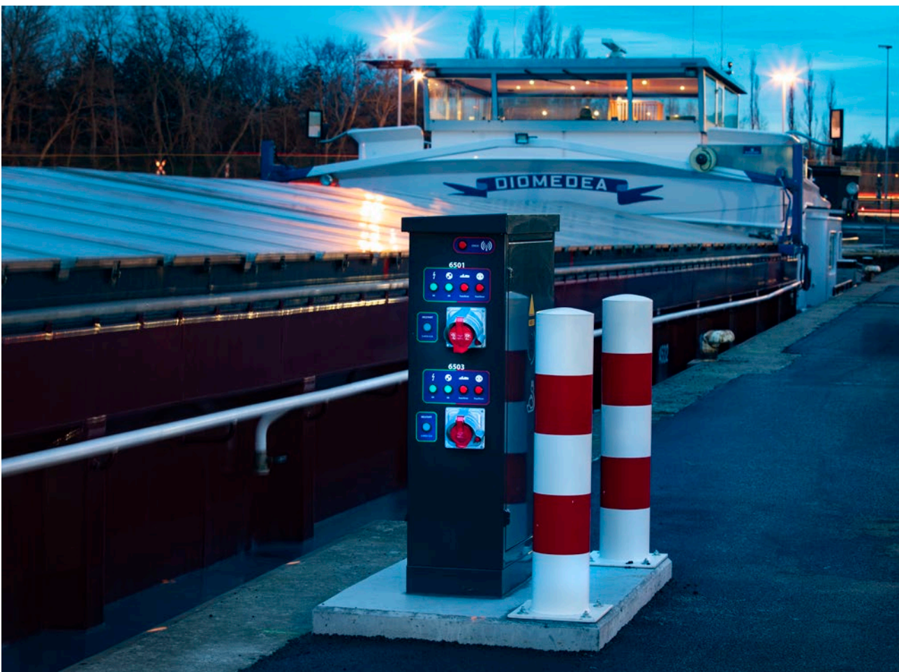
Figure 5: Onshore Power Supply Unit
