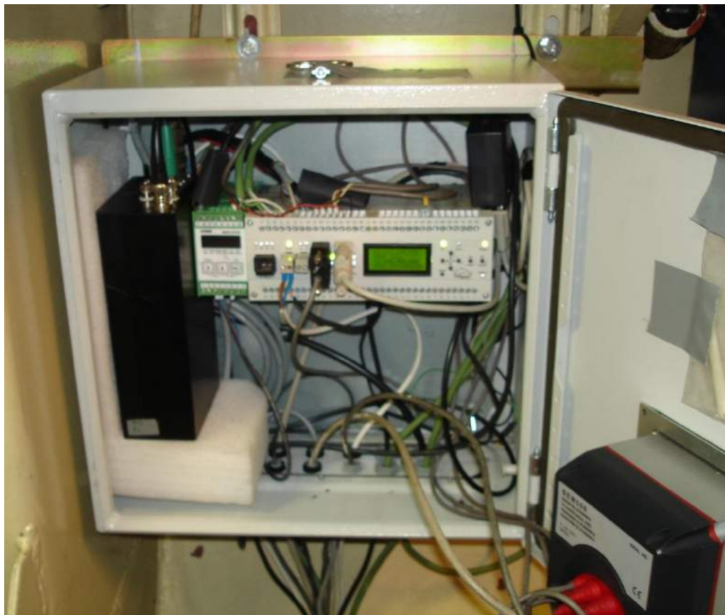
Figure 5: Data Logger for Measurement Data Recording
