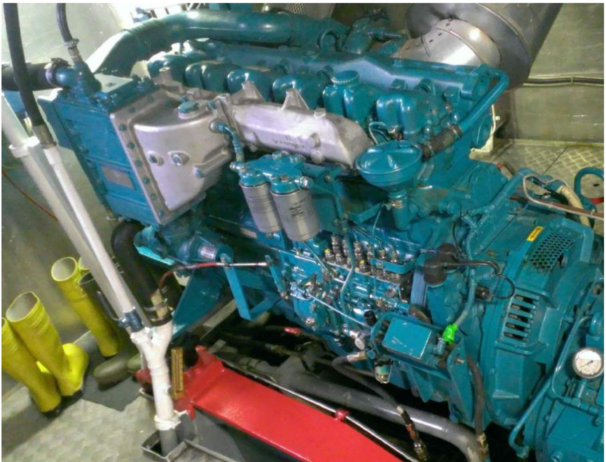
Figure 2: Starboard propulsion engine MAN D2866 LXE43
